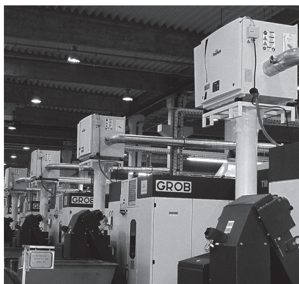
Absolent installation at Premium AEROTEC. Solution: A•mist 100 (one filter unit for each machine)
